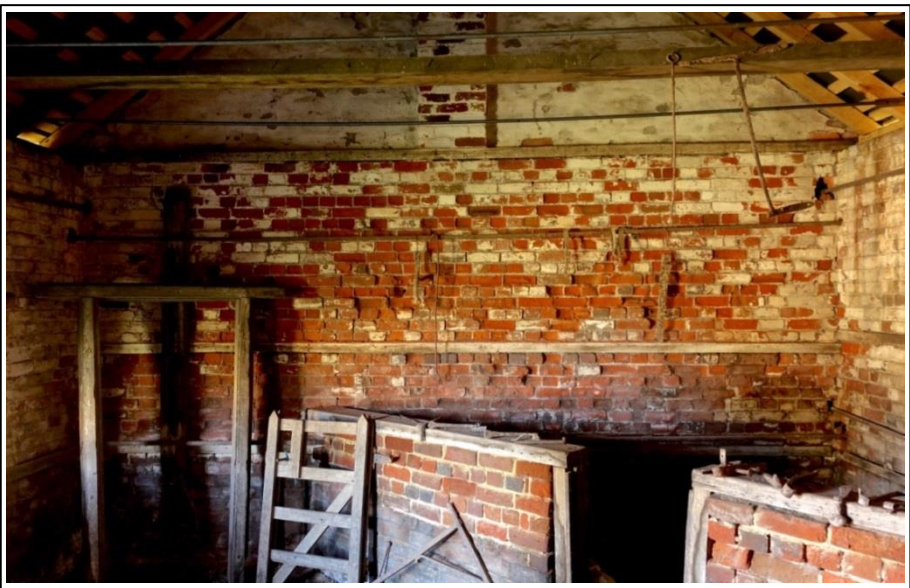
Figure 3: Interior of northwest wall showing extensive decay of low-fired bricks due to salt attack. Early limewash finishes remain on undamaged parts of the wall.
