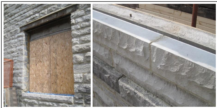
Fig. 4: Representative examples Lannon stone used as a substitute for Platteville stone. Image on the left is a replacement sill and image on the right is a reconstruction of a parapet.
