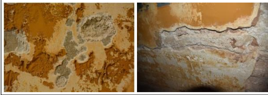
Fig. 2: Exfoliation of inner stucco (left) and middle-layer mortar with salt crystallisation (right)
