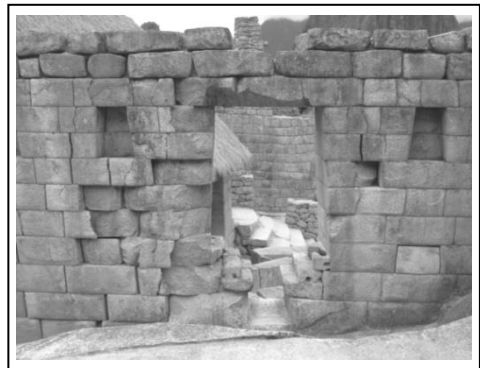
Fig. 4: Severe damage of the northern opening area.
