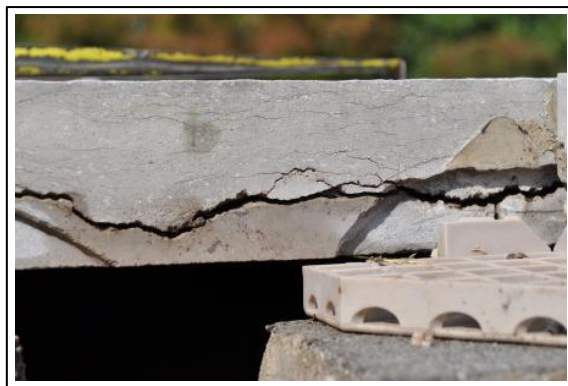
Fig. 7: Typical delaminated Paver.
