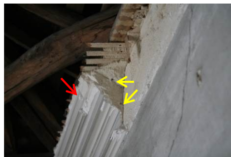
Figure 4.36 - Cross-section of the cornice from where sample ERR3 (red arrow) was taken, with iron rods (yellow arrows)
