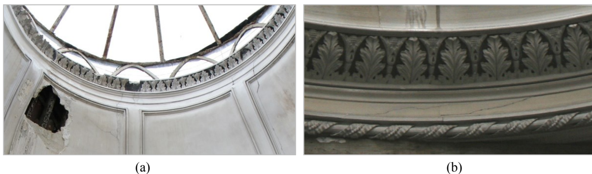
Figure 4.37 - Skylight framed by plaster decorations that have been precast: (a) top frame; (b) bottom frame
