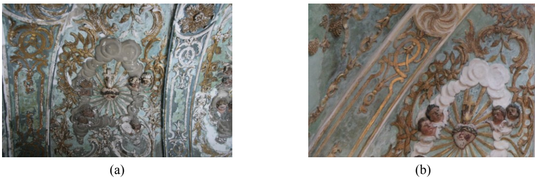
Figure 4.15 - Decorative plasters of the Santissimo Sacramento 's Chapel: (a) before restoration; (b) after restoration
