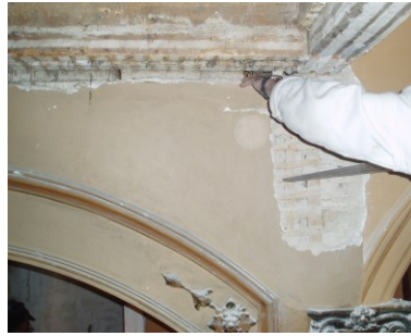
Figure 4.164 - Collection of a sample from the plaster coating of a wall of the Fafe Cine-Theatre building
