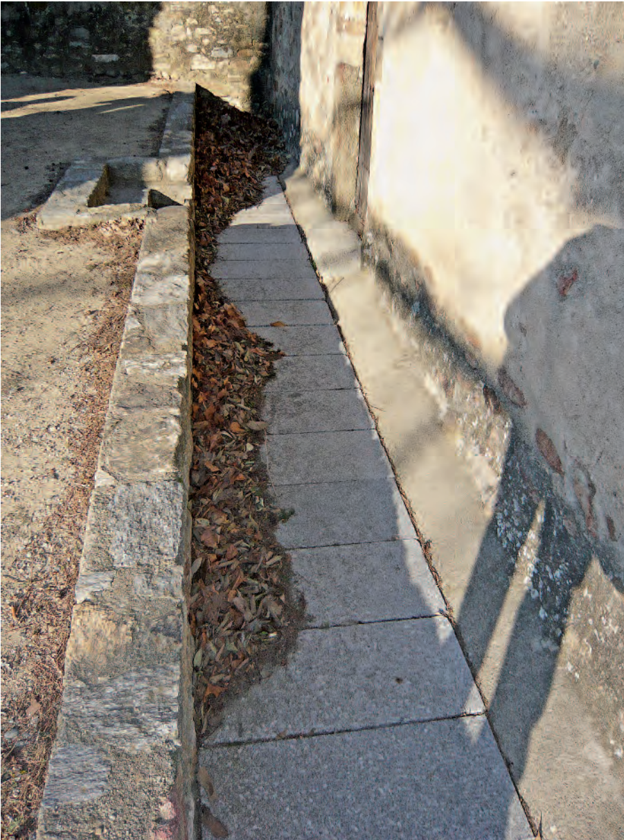
Channel around the Chapel of Saint Martin de Fenollar, Maureillas-Ias-Illas (France), 12th century; Photo: 2012, CICRP (Jean-Marc Vallet)
