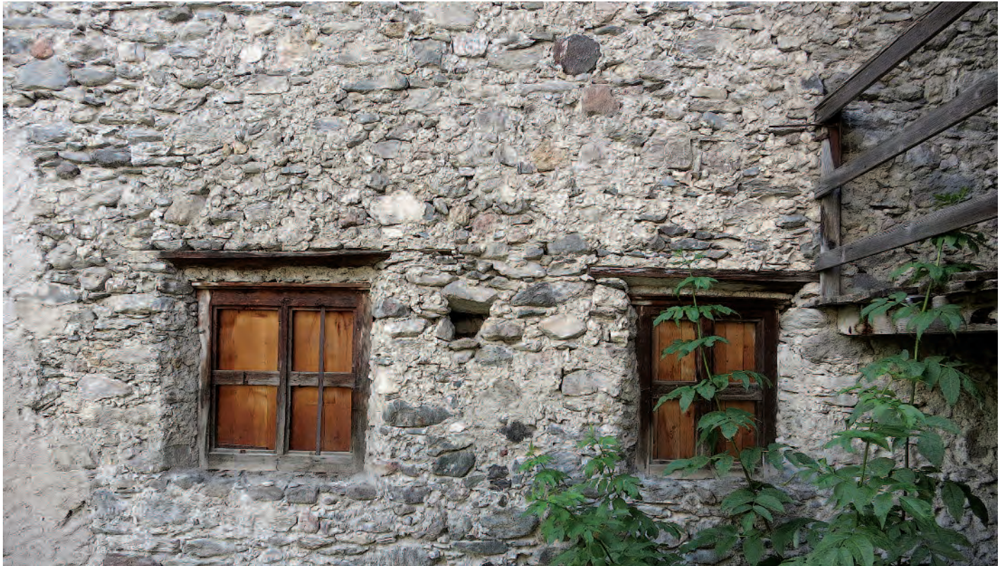
Typical rubble masonry, historic building, Santa Maria Val Müstair (Switzerland); Photo: 2015, HAWK (Angela Weyer)
