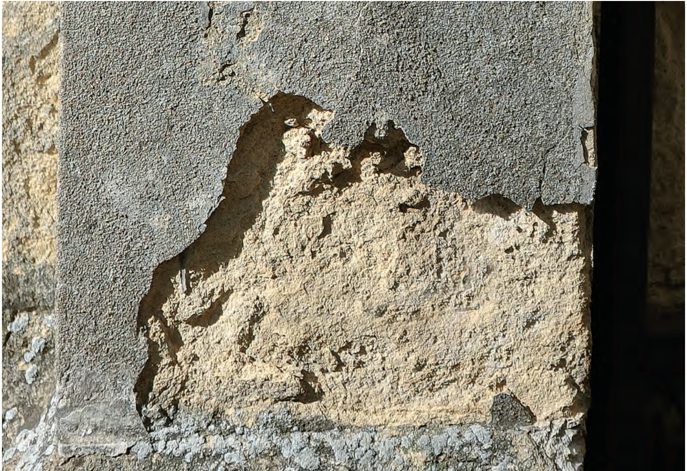
Detachment of plaster, stone fence, Cluj-Napoca (Romania), 20th century; Photo: 2015, UAD (Adrian Rauca)
