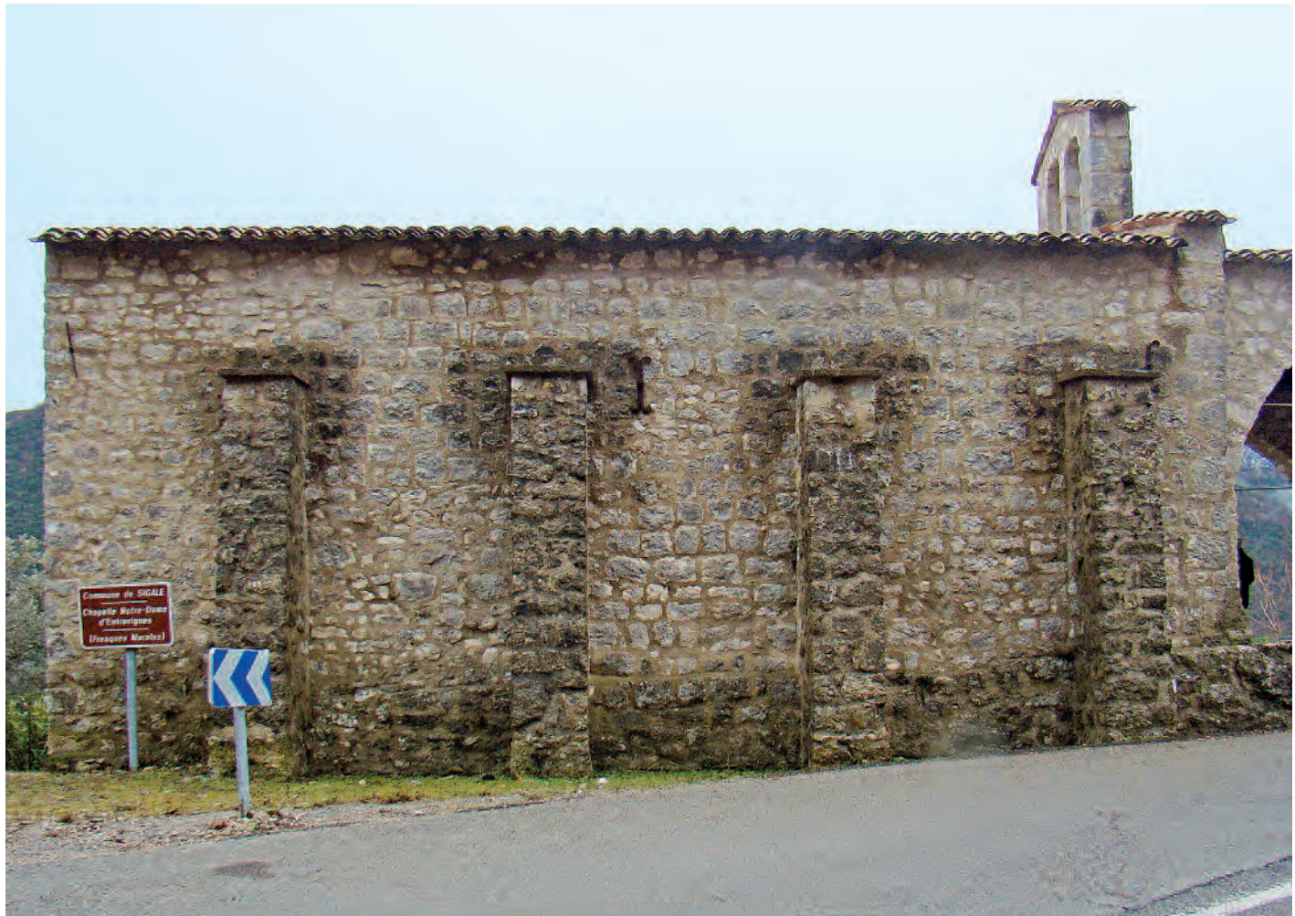
Areas of moisture infiltration are evident as darkened areas, Chapel of Notre-Dame-d'Entrevignes, Sigale (France), 15th century; Photo: 2014, CICRP (Jean-Marc Vallet)
