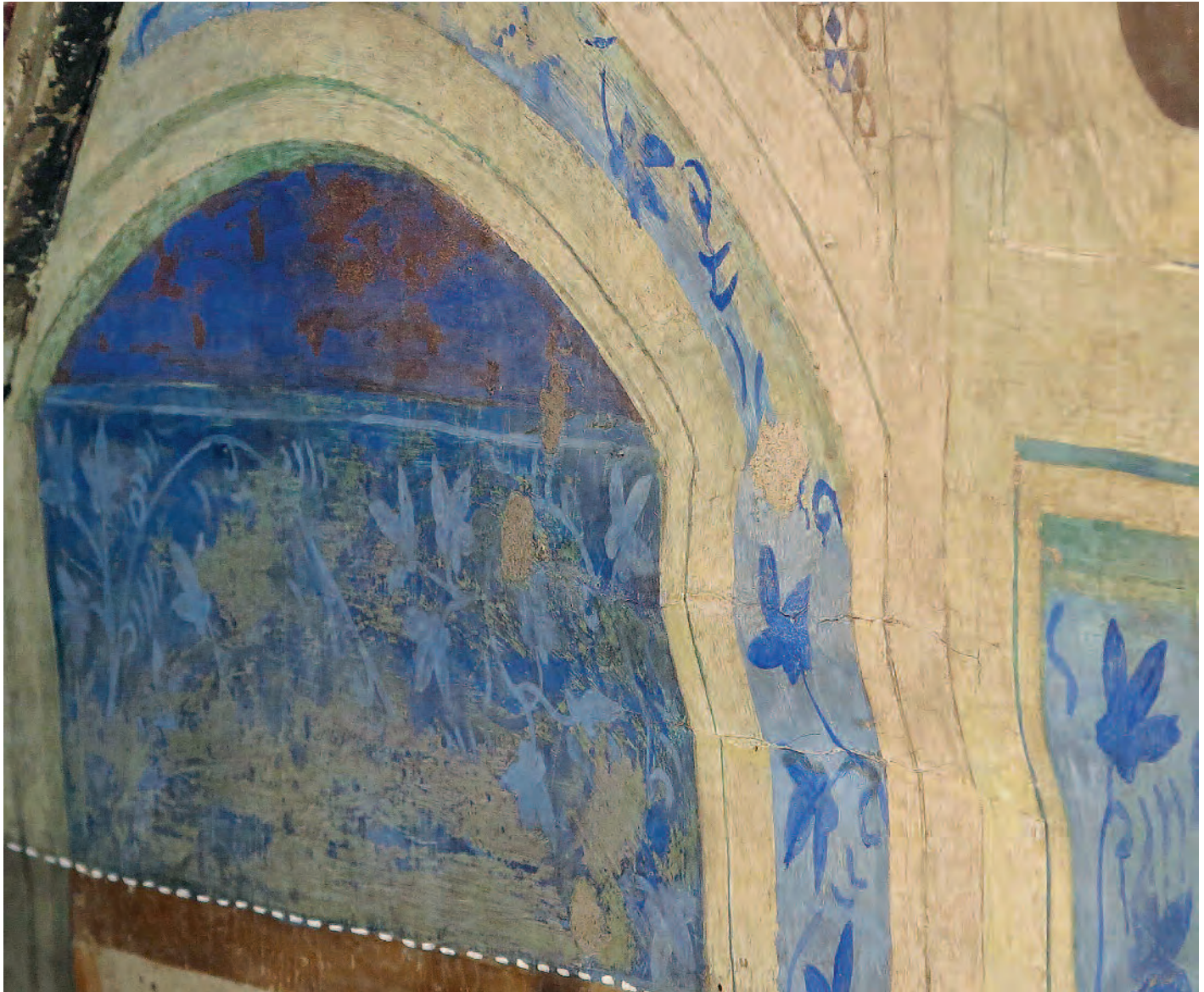
Convex deformation of painted plaster layer, Chapel of Saint-Martial, Palais des Papes, Avignon (France), 14th century; Photo: 2013, CICRP (Jean-Marc Vallet)
