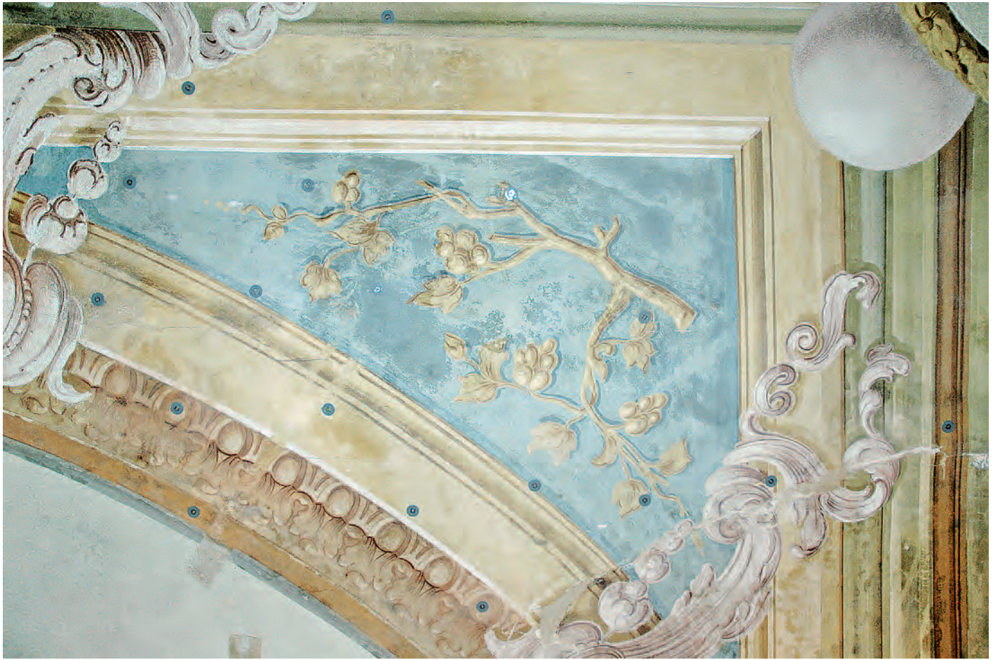
Painting on a ceiling secured by screws, Sorkočević' Palace (Bishop's Palace), Dubrovnik (Croatia), 18th century; Photo: 2008, HRZ (Ivan Srša)
