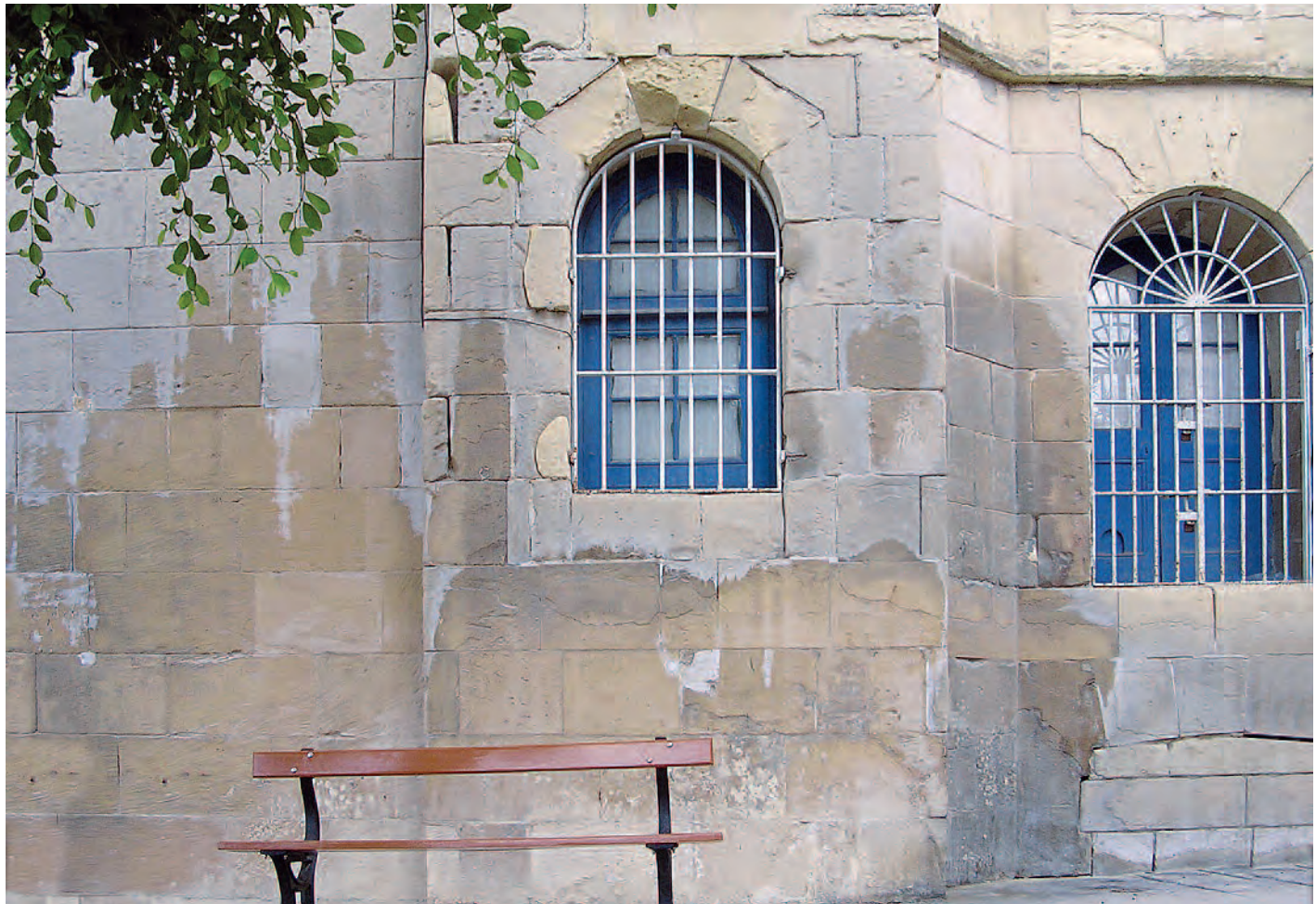
Hygroscopic salts have resulted in a damp patch on a limestone wall (Malta); Photo: 2008, UM (JoAnn Cassar)
