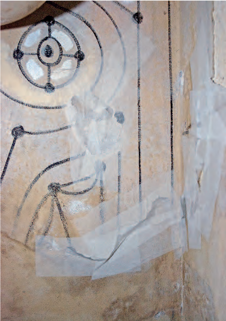
Facing applied to temporarily prevent scaling and delaminated areas from falling, chapel Saint Pierre, Villefranche sur mer (France), painted by Jean Cocteau, 1956/7; Photo: 2008, CICRP (Odile Guillon)
