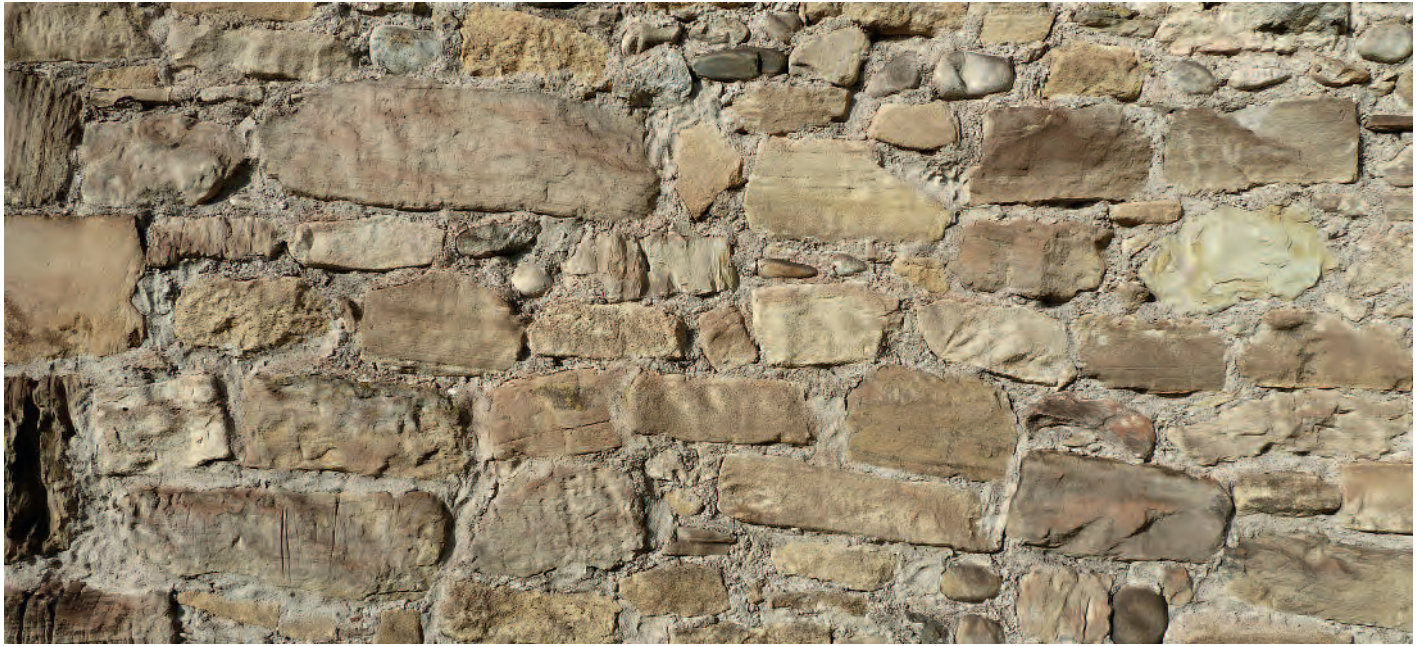
Mixed stone construction, southern façade, Dormition of the Theotokos Church, Strei (Romania), 13th century; Photo: 2015, UAD (Adrian Rauca)
