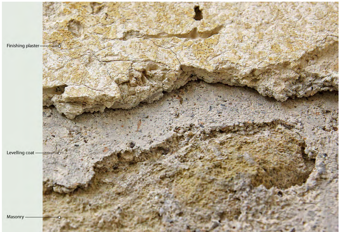
Levelling coat between masonry and finishing plaster (detail), Church of St. John Aliturgetos, Nessebar (Bulgaria), 13/14th century; Photo: 2014 (Stefan Belishki)
