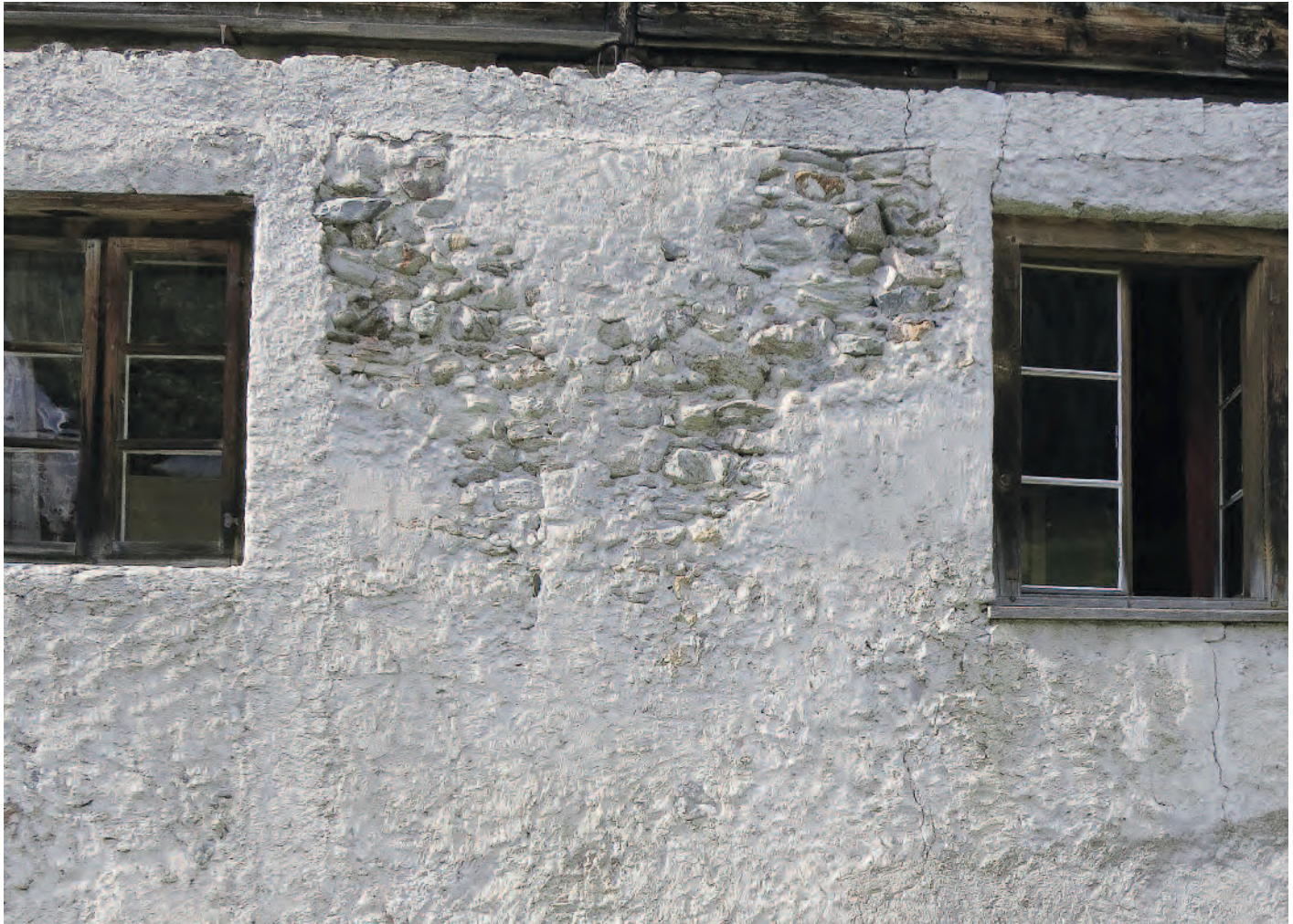
Rendered façade of historic building, Santa Maria Val Müstair (Switzerland); Photo: 2015, HAWK (Angela Weyer)
