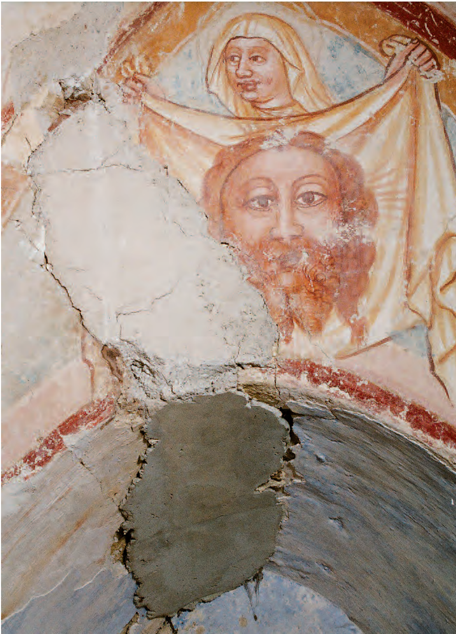
Incorrect plaster application, Chapel of St. John the Baptist, Ivanić Miljanski (Croatia), ca. 1450; Photo: 2002, HRZ (Ivan Srša)
