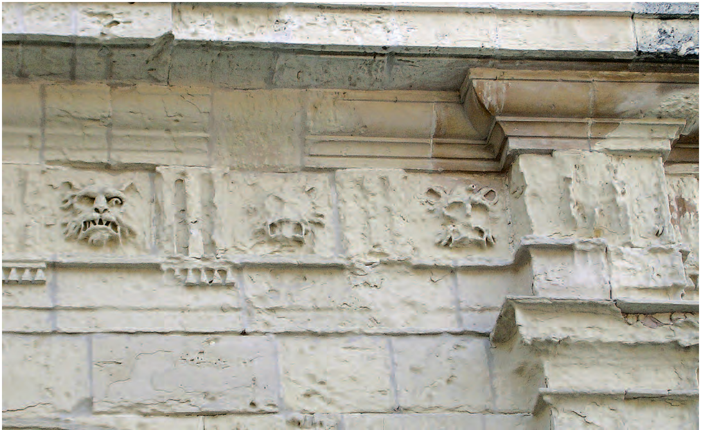
Fluctuating environmental conditions, especially humidity, have led to the deterioration of this salt-laden limestone (part of upper frieze in Globigerina Limestone), Greek's Gate, Mdina (Malta), early 18th century; Photo: 2008, UM (JoAnn Cassar)
