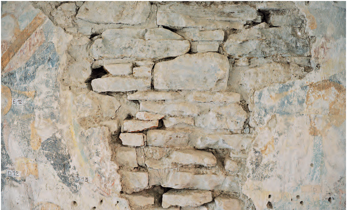
Loss of plaster shows masonry support (detail), Fortified Church in Apold (Romania), 13th century; Photo: 2014, UAD (Adrian Rauca)
