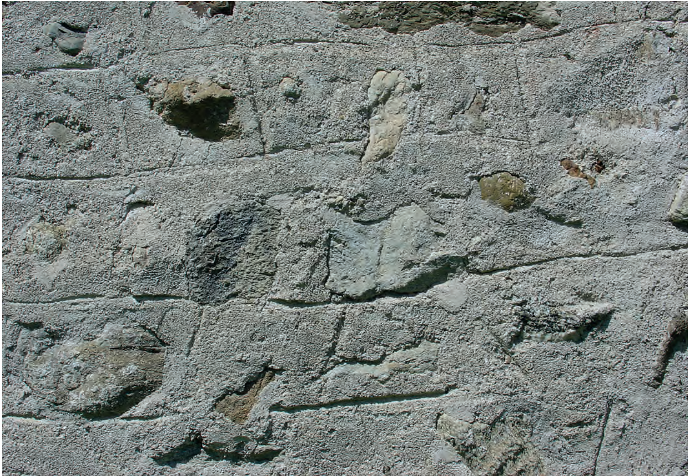
Detail of external wall, Chapel of St. Ulrich, Elmenau (Germany), 12/13th century; Photo: 2004, RPS (Dörthe Jakobs)
