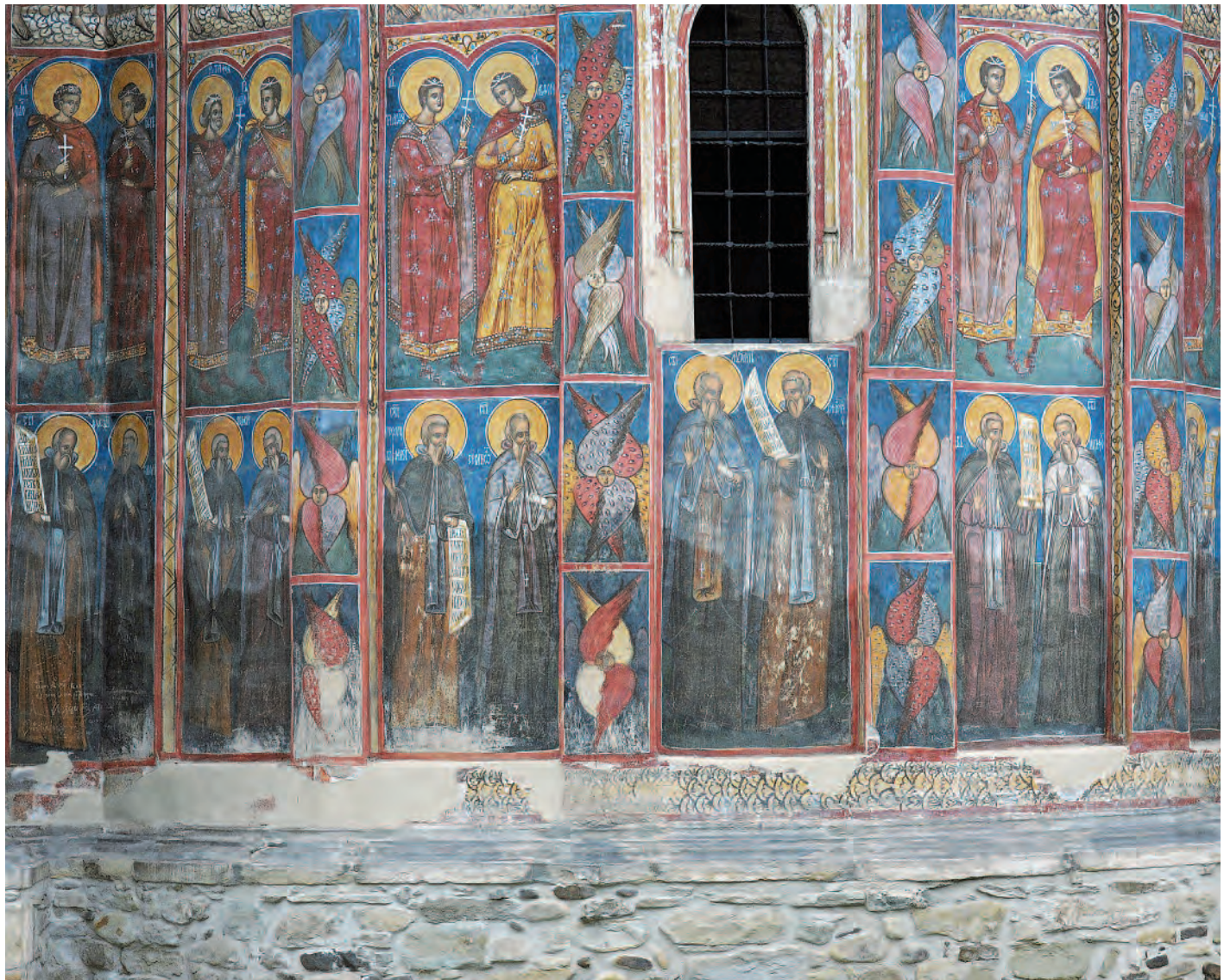
Rising damp visible as colour saturation, Moldovița Monastery (Romania), 1532; Photo: 2003, UAD (Theo-Sandu Mureșan)
