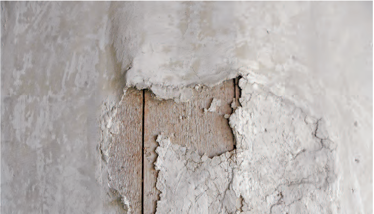
Fragmentary whitewash on damaged plaster layer, Çeyrekçiller House, Safranbolu (Turkey), 19th century; Photo: 2012, KBU (Aysun Özköse)
