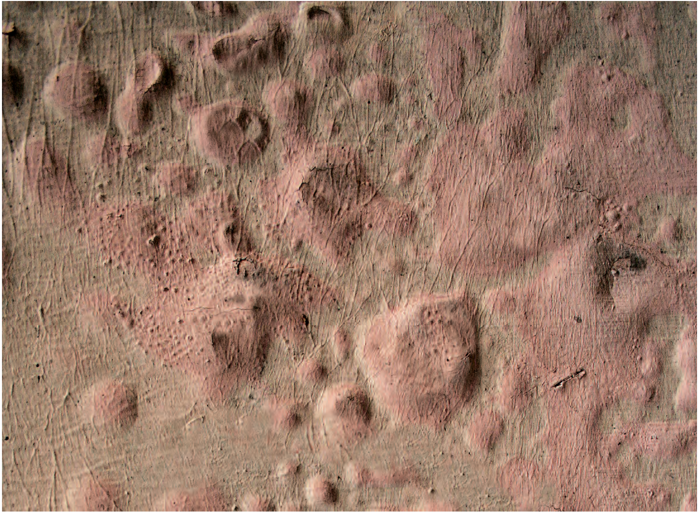
Paint layer showing bulges, Secco wall painting, Cluj-Napoca (Romania), 19th century; Photo: 2015, UAD (Adrian Rauca)
