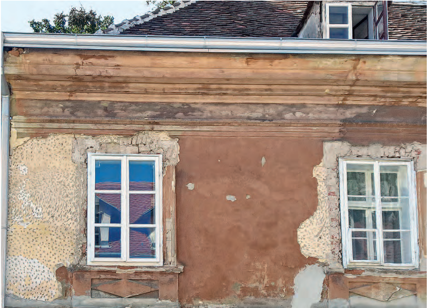
Losses of the top render layer allow a view of the layer beneath, showing traces of keying by hammering, historic building, Zagreb (Croatia); Photo: 2015, (Roland Lenz)
