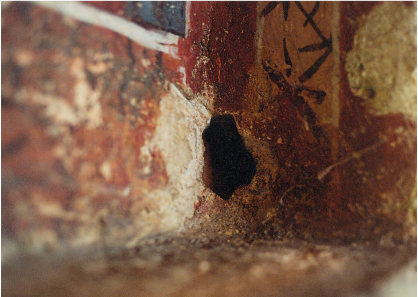
Deep hole in external wall painting, Moldovița Monastery (Romania), 1532; Photo: 1993, UAD (Theo-Sandu Mureșan)
