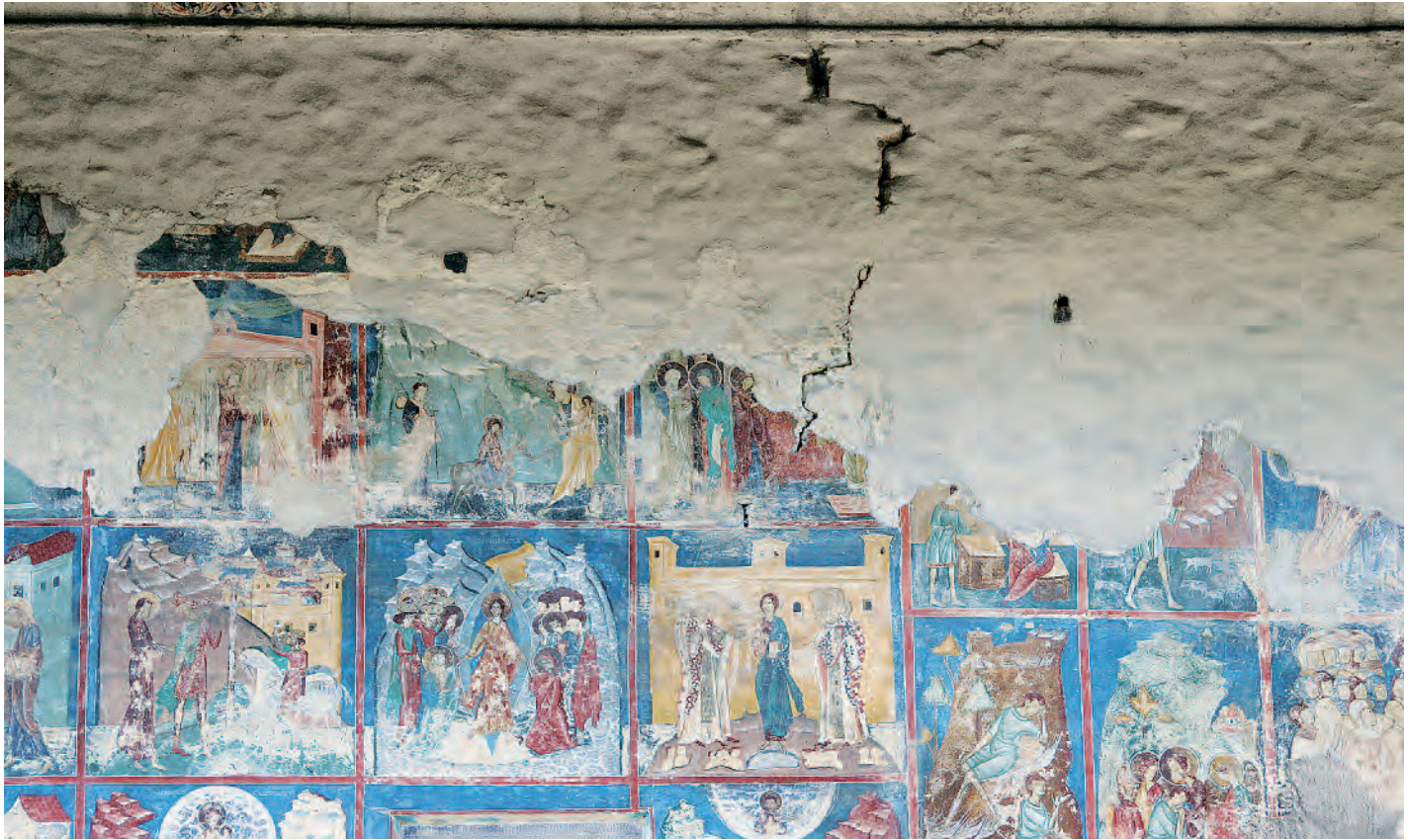
Crack caused by structural movement of a building, Arbore Church (Romania), 1502; Photo: 2012, UAD (Adrian Rauca)
