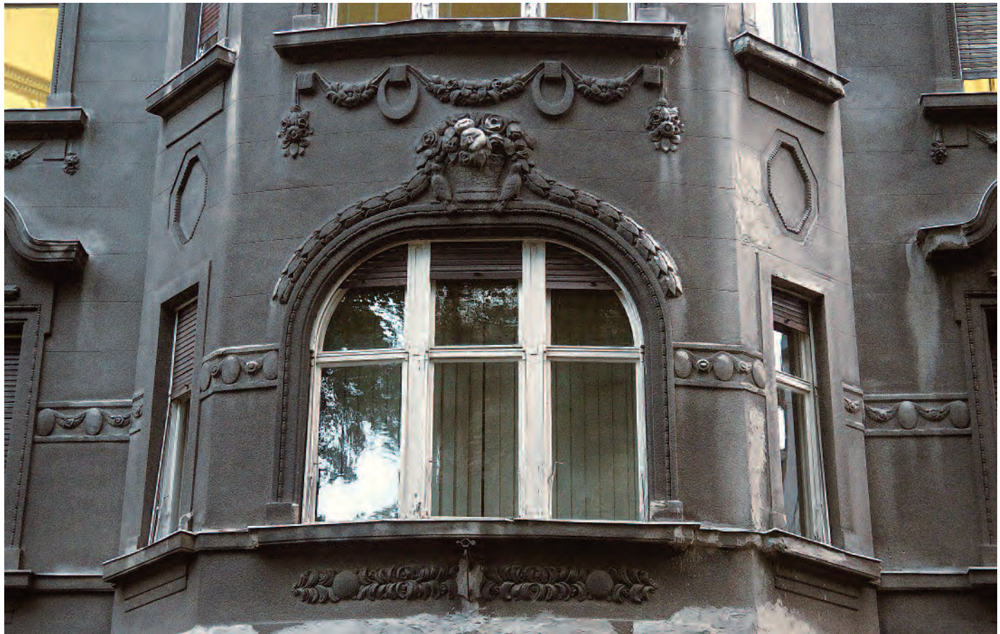
Darkened render on a façade, private building, Zagreb (Croatia), early 20th century; Photo: 2015, (Stefan Belishki)
