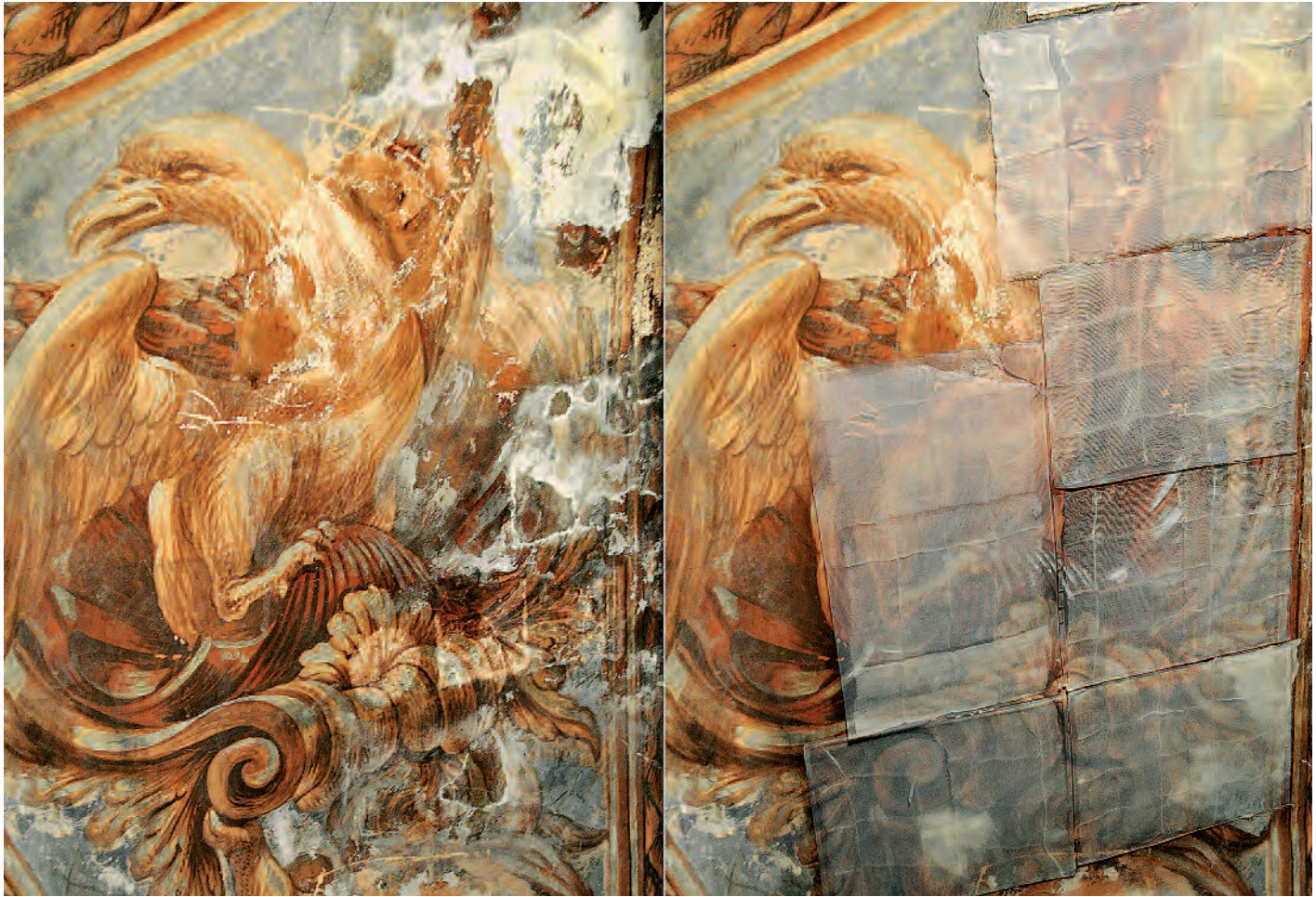
Salt efflorescence on a wall painting (left), example of salt reduction (right) on a wall painting by Antonio A. Palomino/ Guillo, Church of Santos Juanes, Valencia (Spain), 1698-1700; Photo: 2011, UPV
