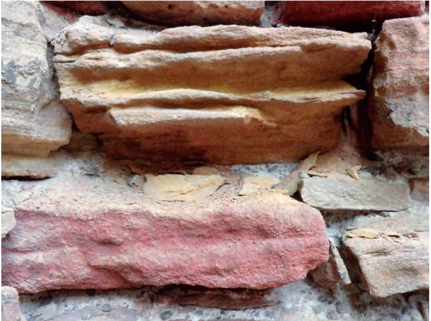
Loss of material caused by wind erosion, Dominikanerkirche, Colmar (France), 1289–1346; Photo: 2015, RPS (Dörthe Jakobs)
