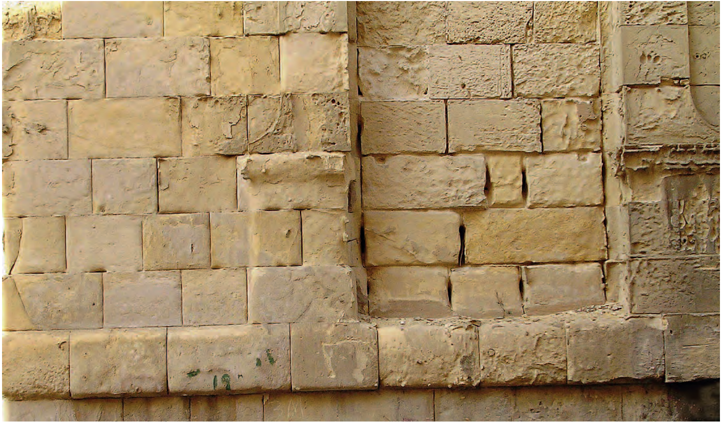
Wet-dry cycles, in the presence of soluble salts, lead to severe deterioration in porous limestone (Malta); Photo: 2008, UM (JoAnn Cassar)
