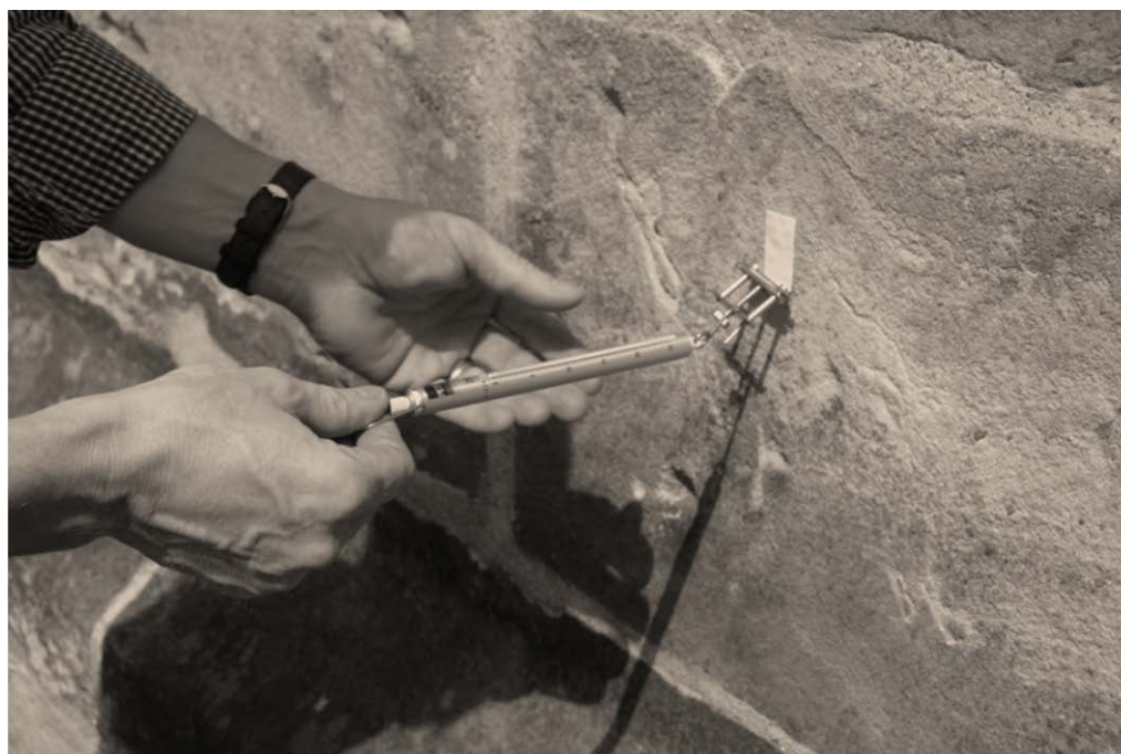
Figure 4. Power Strip Test, Görlitz, Heiliges Grab, Germany (photo Christoph Franzen)
