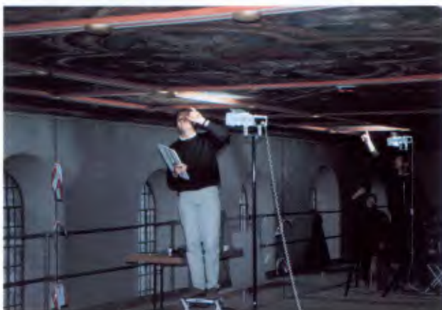
Figure 8. Germany, Protestant church of St Michael, Romanesque ceiling. The in situ mapping of damage.
