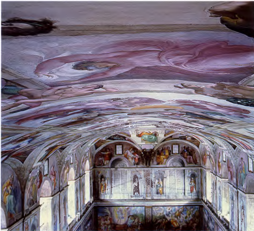
Figure 4. View of the irregular curvature of the vault of the Sistine Chapel.
