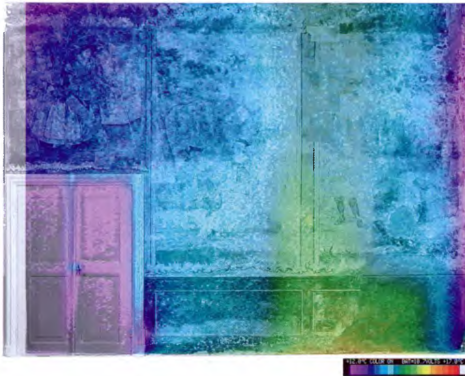
Figure 13. Manor house Altenkamp, entrance hall, image map of the south wall, overlaid with thermo image. The thermo image consists of four images. Radiation between 8 and 14 \mu\text{m} reflected by the object was registered. The picture shows cold areas on the edges of the walls (connection with exterior walls or non-heated adjoining rooms). The warmer (green) area in the middle indicates that warmth is sucked off through an open fireplace in the adjoining room.
