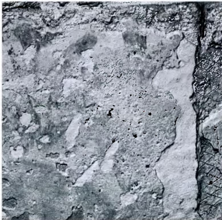
Figure 15. Scan (orthoprojection) of damaged wall.
